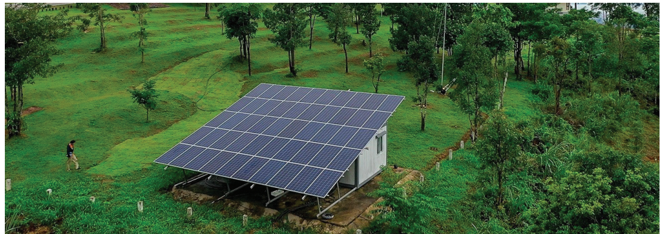
Movable PV system at Phu Lean Kha National Park, Chaiyaphum province
