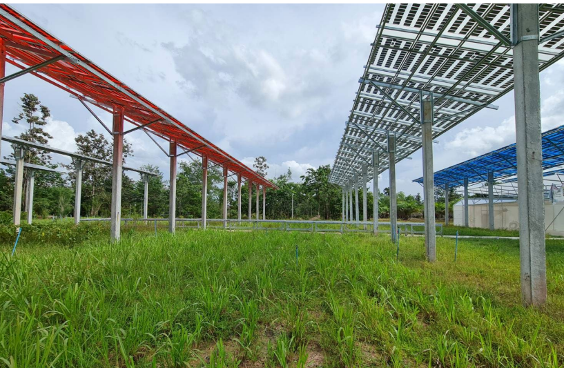
Figure 2.12 Typical microgrid system with a 28 kWp installed capacity combined with a 21.3 kWh Battery Energy Storage System (BESS), integrated with farming in Ubon Ratchathani Province, and operated by NSTDA.
