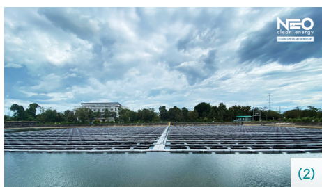
(2) 806 kWp floating PV system in khao Yoi, Phetchaburi province.
