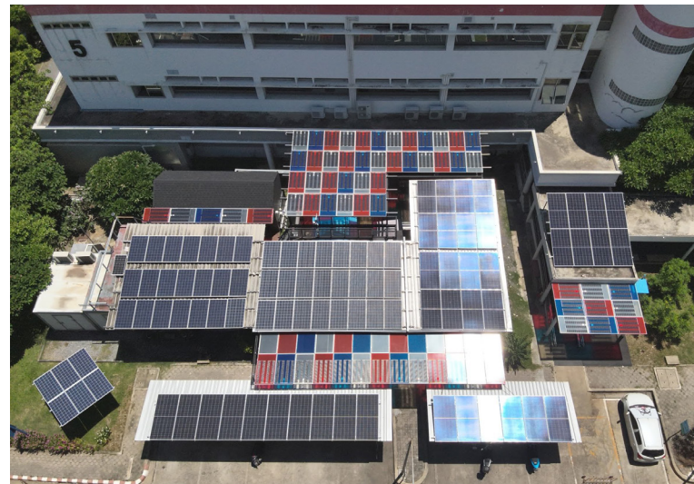
Figure 2.13 PV microgrid at NECTEC pilot plant in Khlong Luang district, Pathum Thani province.
