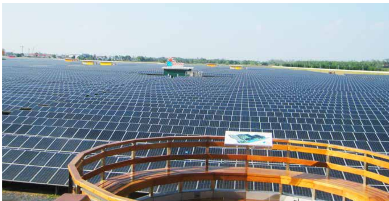
Fig. 2.3 : 35.64 Mwp at Bang Pa-In district, Ayutthaya, which commenced commercial operation in July 2012 (Photo: Bangchak Solar Energy Co., Ltd.)
