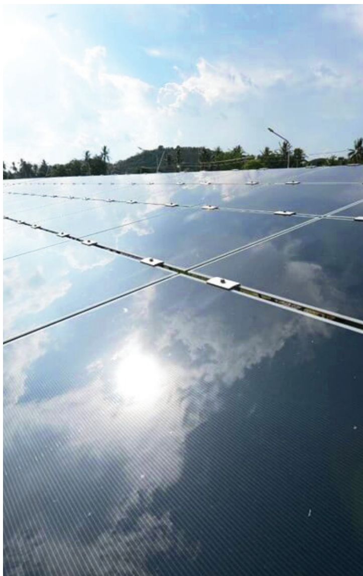
Thap Sakae PV power plant at ThapSakae District, Prachuap Khiri Khan Province
