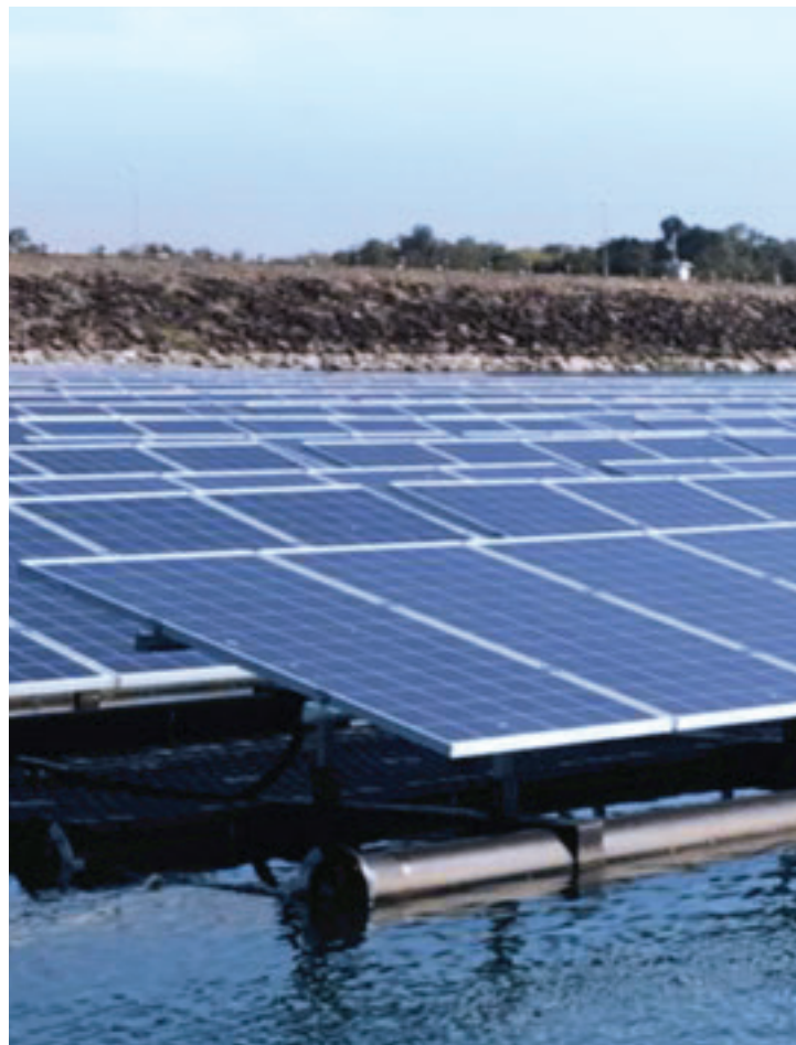
Floating PV system at Sirindhorn Dam, Ubonratchathani Province
