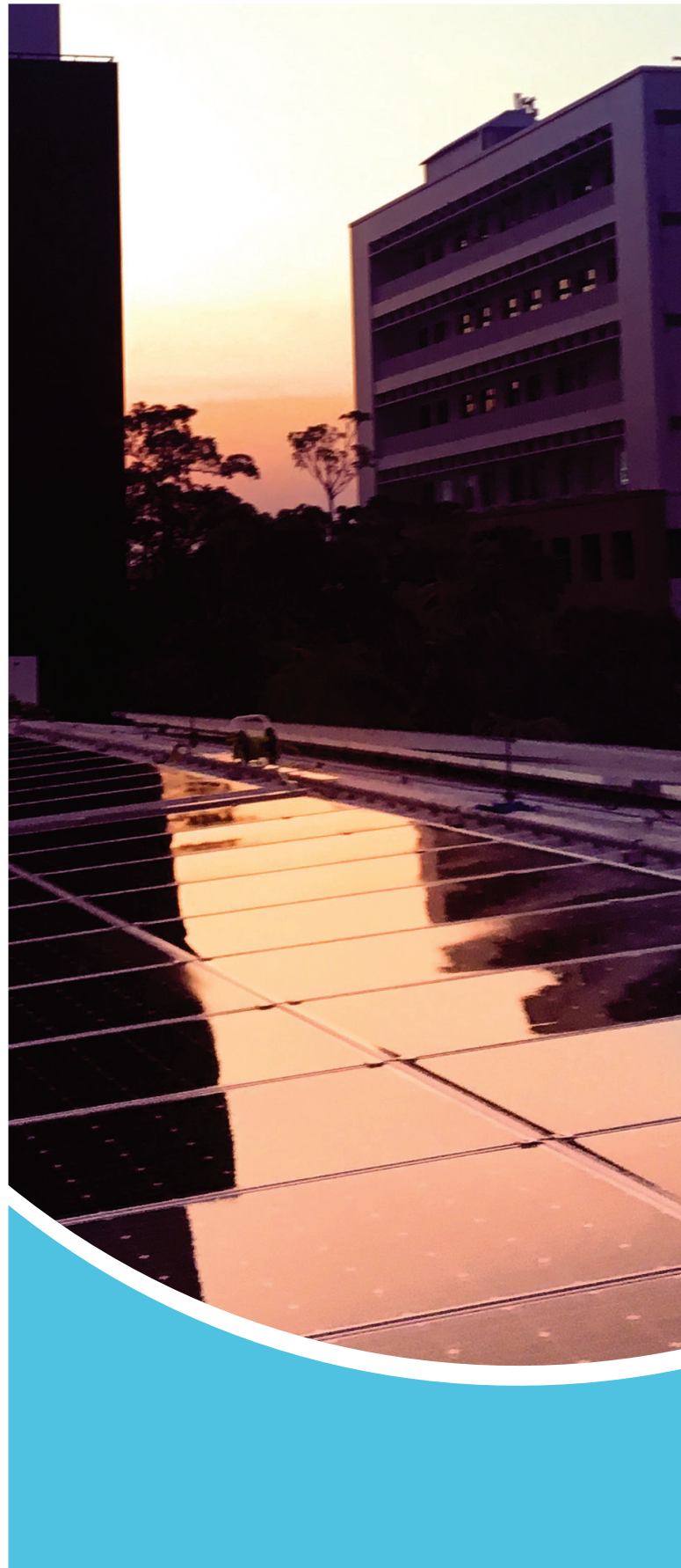
Rooftop PV system at KMUTT Bang Khun Thian district, Bangkok
