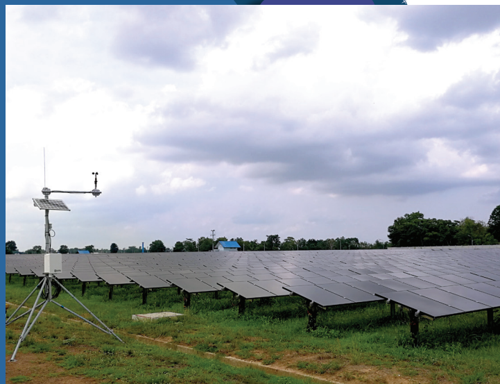
Bangkhenchai PV power plant at Pak Thong Chai district, Nakhon Ratchasima Province
